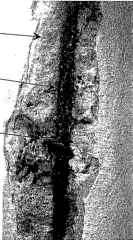
STAGE ADDITION CONCRETE COLUMN SPALLING AND REINFORCEMENT CORROSION
